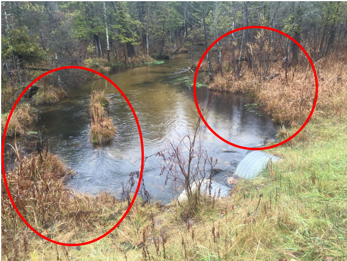
Figure 6. The upstream side of the Finch Creek Rd Crossing of Finch Creek. Backwash eddies causing stream bank widening and increased sediment load
