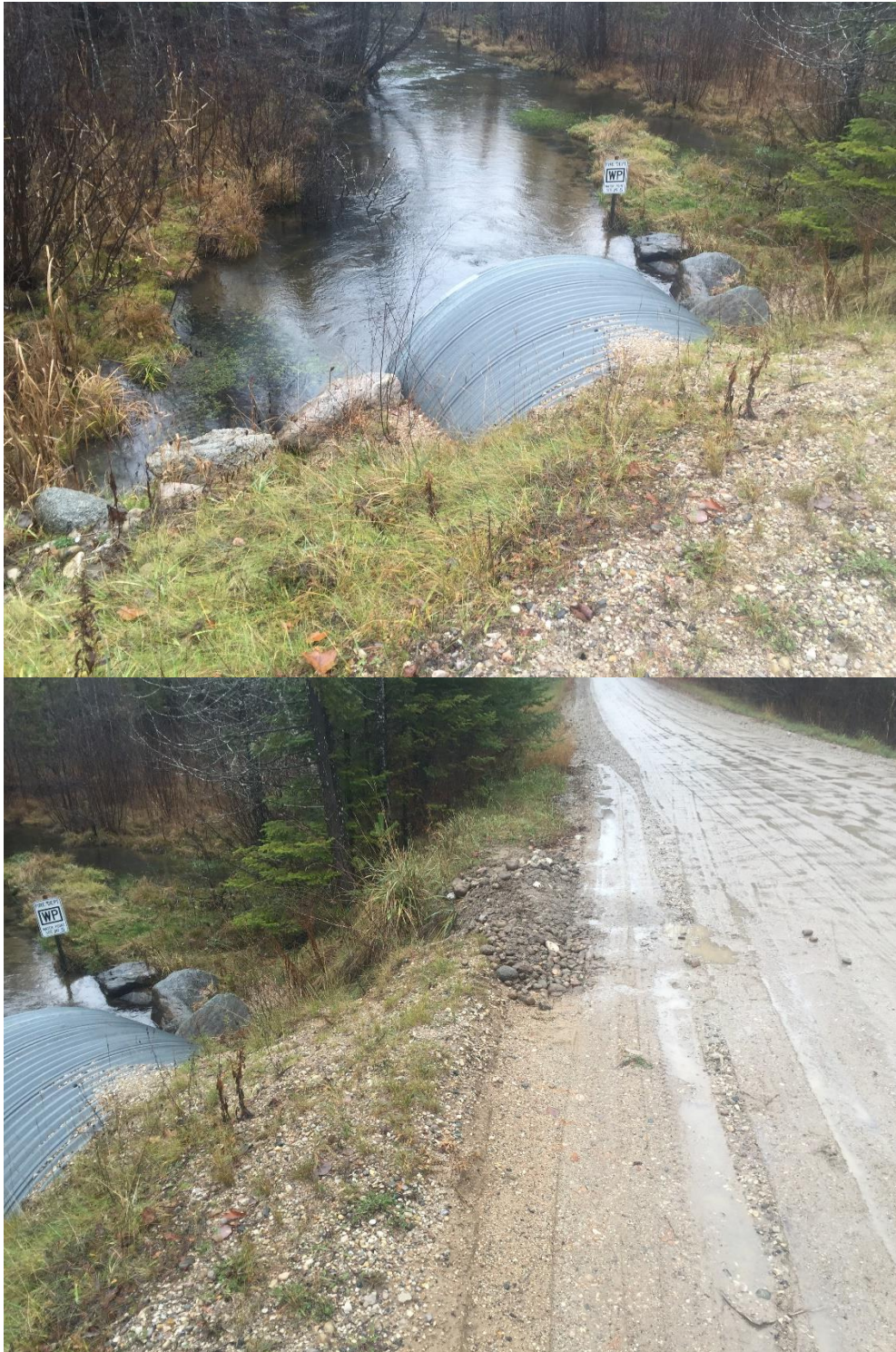
Figure 3. The downstream side of the Tyler road crossing. In the second photo you can see where the road had washed out and was “fixed” with more stone. These wash out events can increase sediments loads far greater than typical sediment loads of poor quality road crossings
