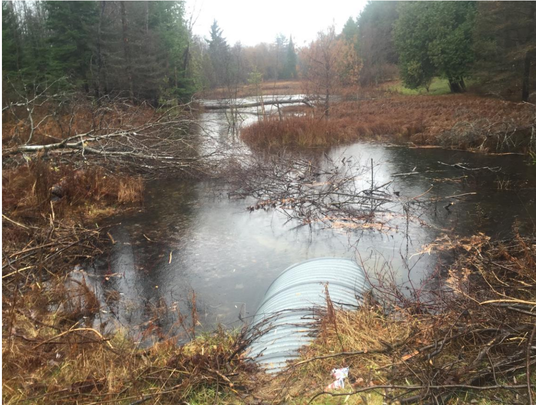
Figure 5. Downstream side of the Grass River Rd crossing. Again, the river is starting to push into its flood plain during the recent rain event
