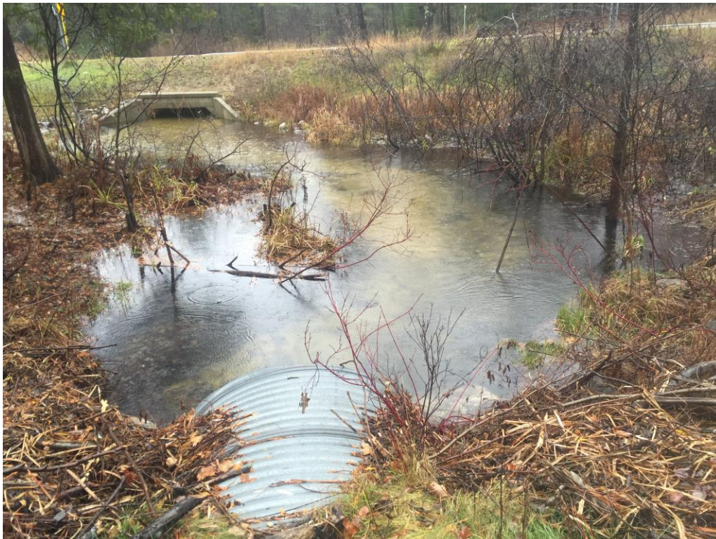
Figure 4. Upstream side of the Grass River Rd crossing. The farthest structure upstream is the M88 Crossing of Shanty Creek. This picture was also taken during a rain event and the stream is pushing into its flood plain
