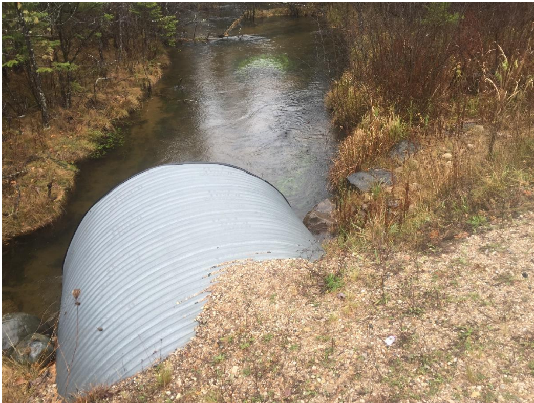
Figure 2. The upstream side of the Tyler road crossing on Cold Creek. You can see the culvert with no “bank” to prevent road material from washing into the stream. This culvert is likely undersized causing bank erosion and stream widening
